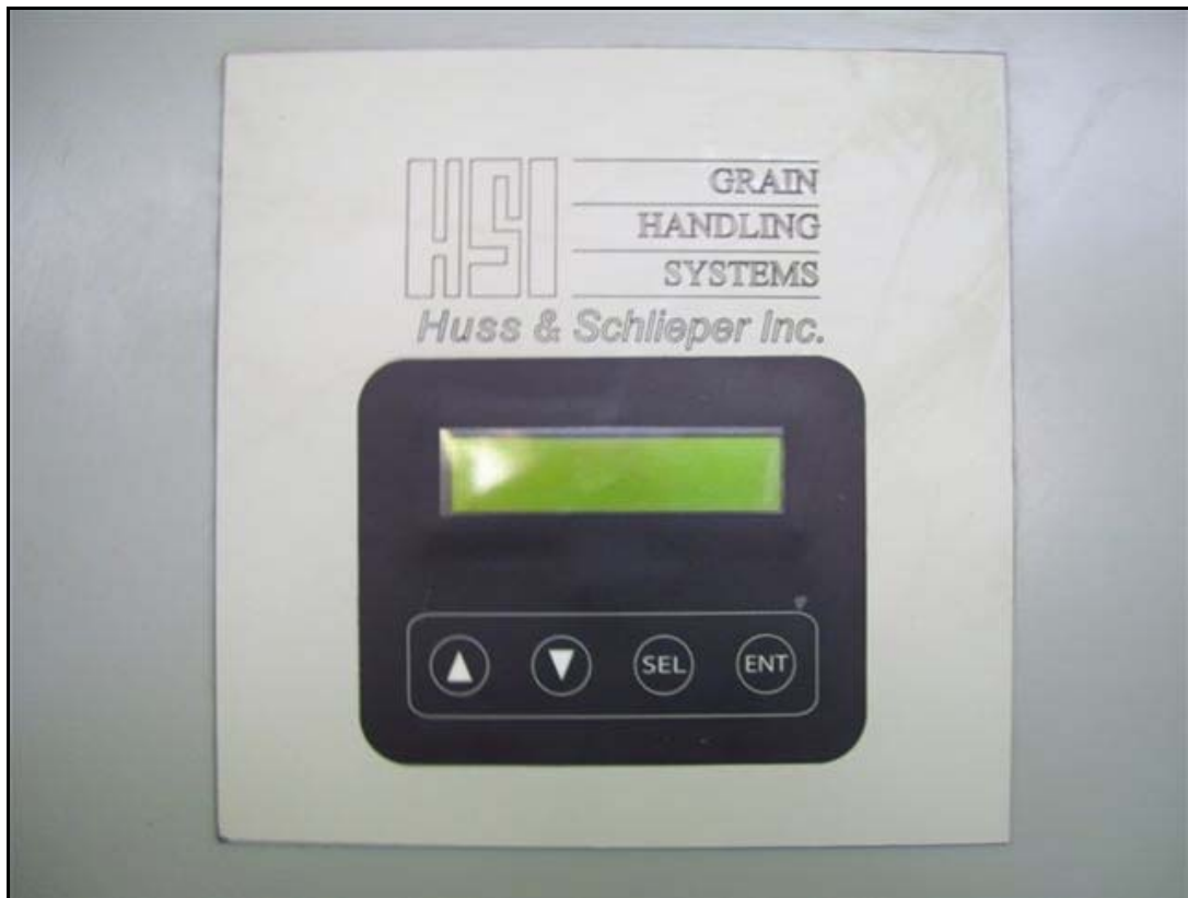
Figure 3.4 Control Panel Close-Up
