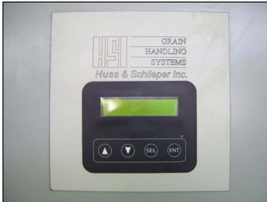
Figure 4.2 Control Panel Close-Up
